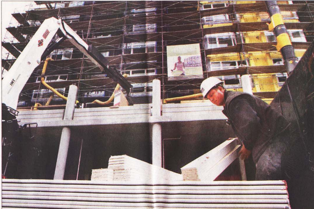
Having just piloted a load of drywall up to the second floor, John Robinson readies another at the soon-to-be completed Ellipse apartment building in the University District. The building has been sold to investors outside the Seattle area.
